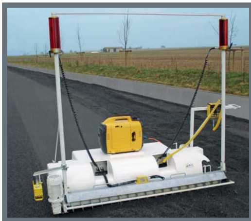
» Minigrader used in the construction of a bikeway — equipped with a MOBA Dual-Laser-matic
