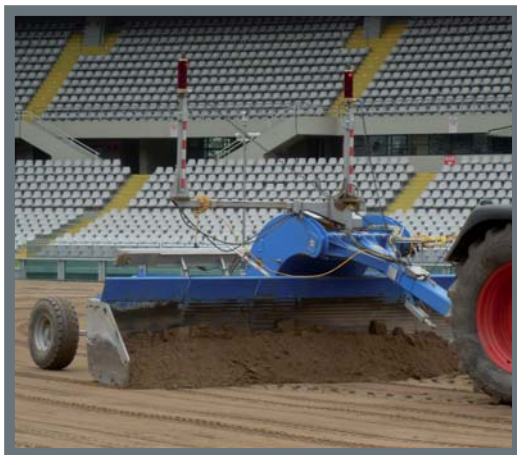
» Stadio delle Alpi – MOBA Dual-Laser-matic used for leveling works in the soccer stadium of AC Turin (Italy)
